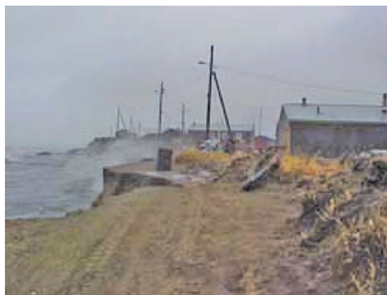
Figure 1. Shishmaref, AK. Erosion from winter storm surges required the village to be relocated. Source: Shishmaref Erosion & Relocation Coalition
